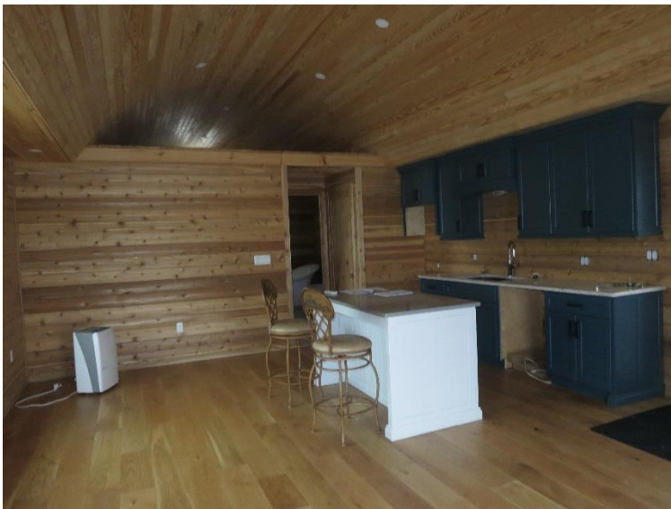
Photo 15: Existing accessory structure – proposed secondary dwelling unit – interior view of kitchen, living area and bathroom
