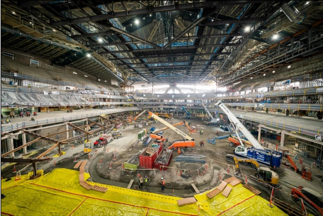
Figure 2: Climate Pledge Arena being constructed underground to increase the capacity of the original Washington State Coliseum. Source: Obando, 2021
