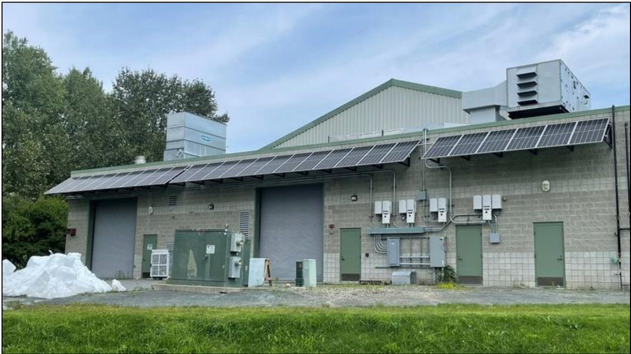
Figure 6: The south-facing roof of Woodstock Union Arena consists of 211 400-watt solar panels angled to optimize solar absorption. Source: Whitchruch, 2021
