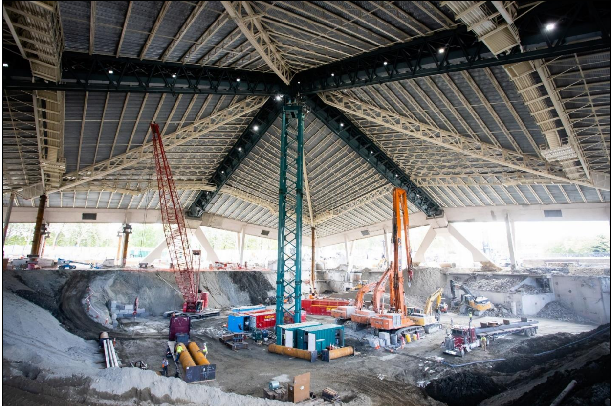
Figure 1: Original Washington State Coliseum roof being supported while the Climate Pledge Arena is built below it. Source: Obando, 2021
