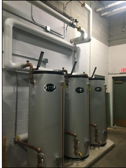
Figure 7: Heat recovery system storage tanks refurbished from the original refrigeration system at Woodstock Union Arena. Source: Whitchruch, 2021
