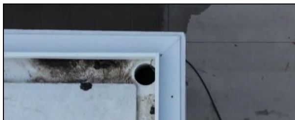
Figure 4: An aerial view of one of the rainwater ducts on Climate Pledge Arena.
