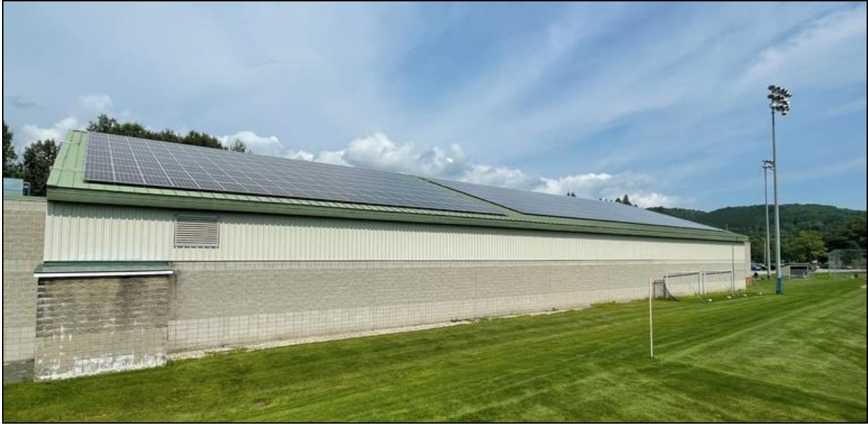
Figure 5: East facing roof of Woodstock Union Arena consisting of 644 430-watt solar panels. Source: Whitchurch, 2021
