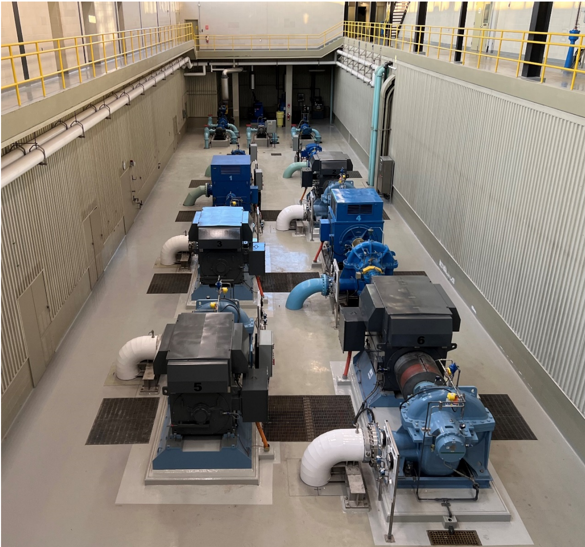
Figure 4: High Lift Pumping Station (September 2022); Original Pumps #1 and #4; New Pumps #2, #3, #5, #6.
