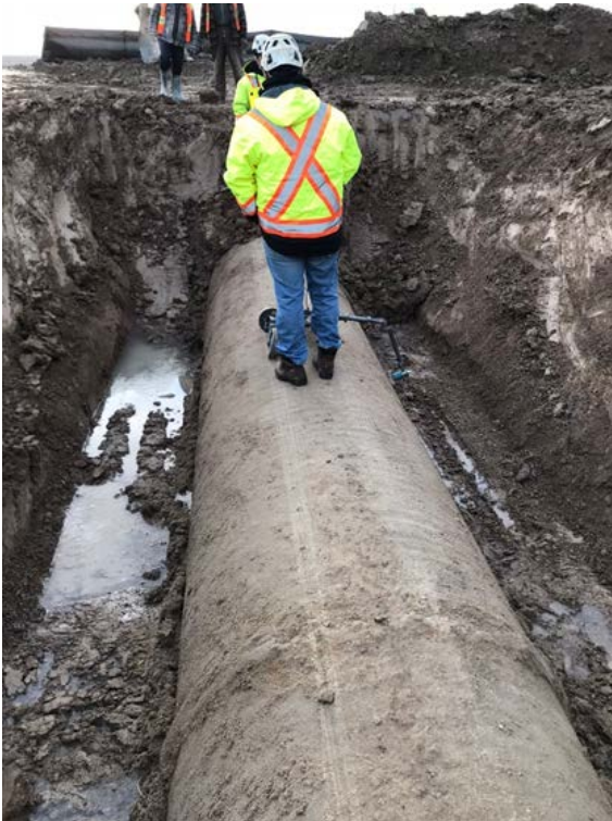
Figure 5: Pure Technologies performing an external electromagnetic verification to confirm the location of distressed pipe #1-162
