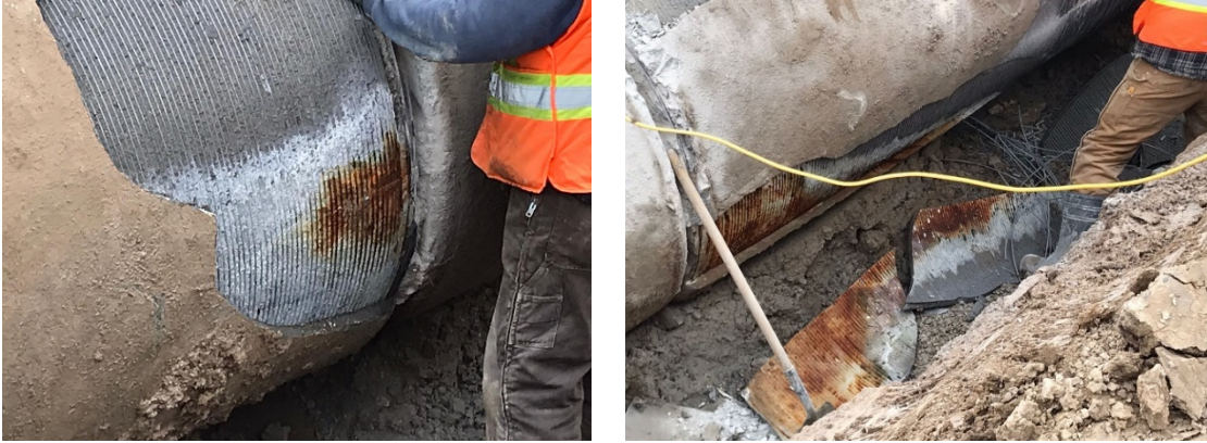
Figures 6a and 6b: Distressed pipe #1-162 showing significant deterioration and wire breaks
