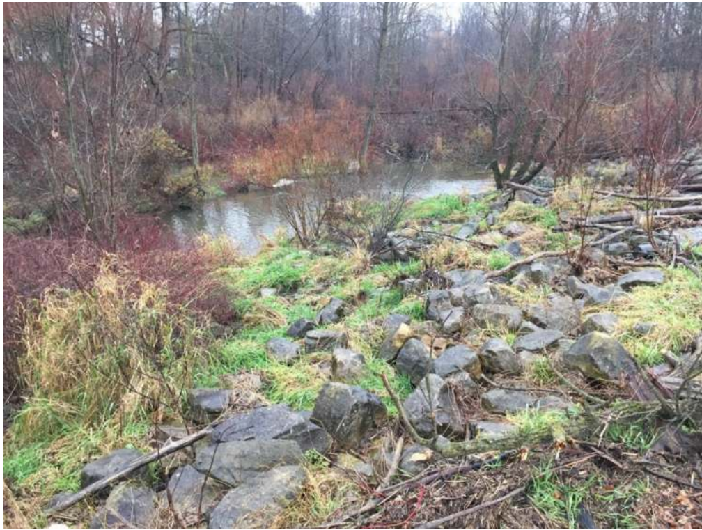
Photo 2: Large sloping armour stone placement on downstream side of sheet pile dam. Sydenham River downstream of dam visible in background.
